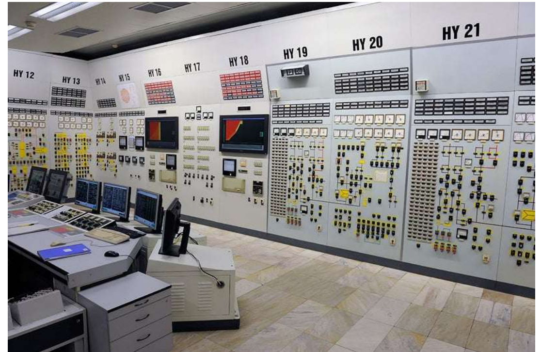
SMR control panel (Power Technology)
