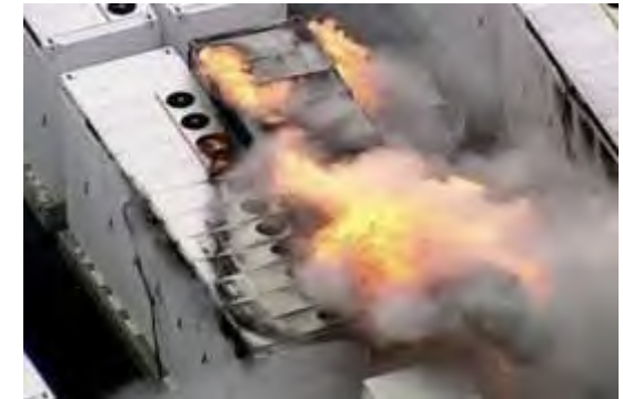
Tesla Megapack Fire, Geelong, Australia, July 2021
