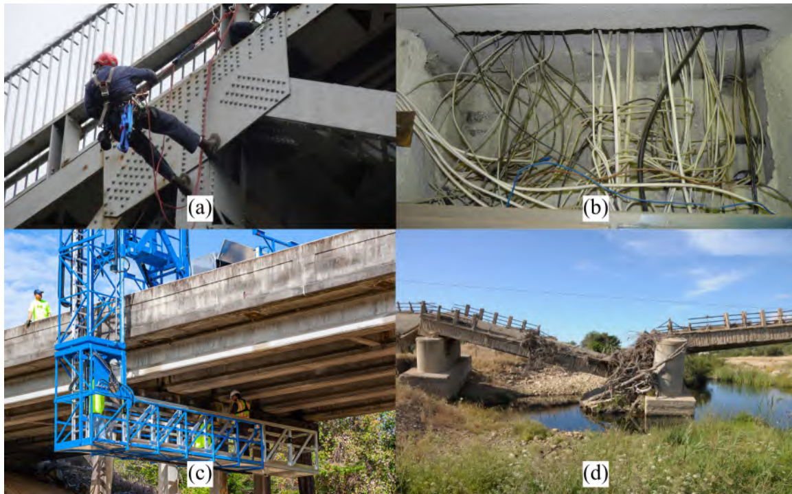
Figure 1.1: (a) A suspended bridge inspector on a riveted steel bridge [34], (b) Wiring through a concrete shaft [11], (c) Dedicated crane for bridge inspection [10], (d) Bridge collapse after flooding event [25].
