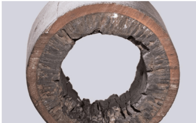
Figure 1.6 Scale buildup in a pipe section, restricting flow and potentially impacting the efficiency of the cooling system [17].
