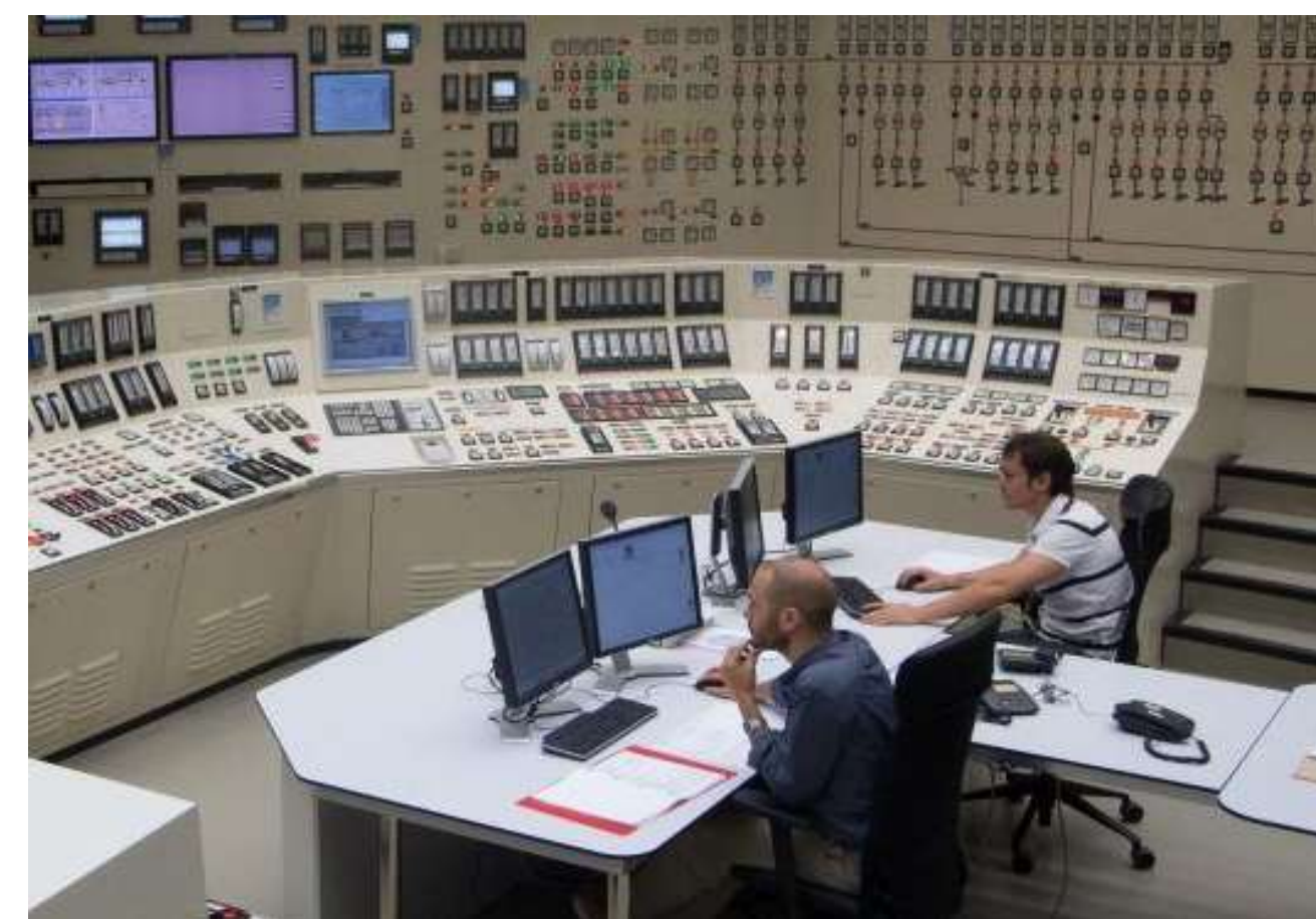
Figure depicts a typical nuclear control panel, where no option for remote operations and digital twin testing is present.
