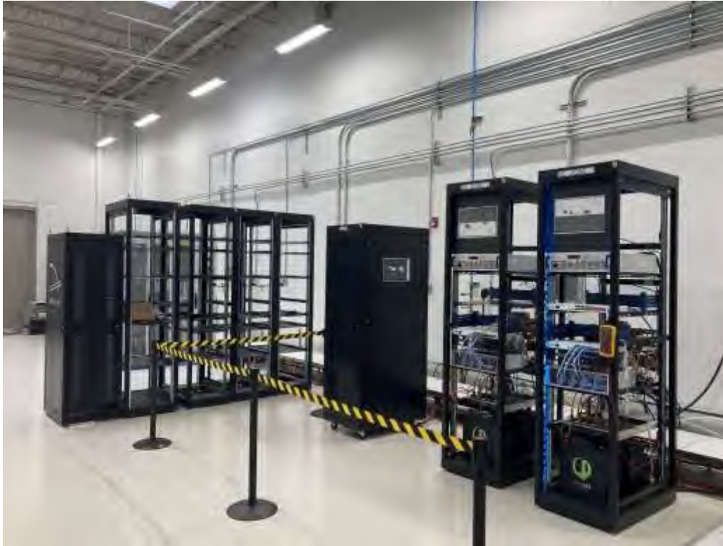
Two DC zone cabinets, 10 bus system, (AC cabinets not yet complete)
